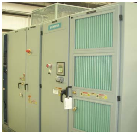
Figure 8-1: Front View of Cell Door Filter during Normal Operation
