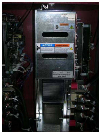
Figure 8-5: Typical 100A Power Cell
